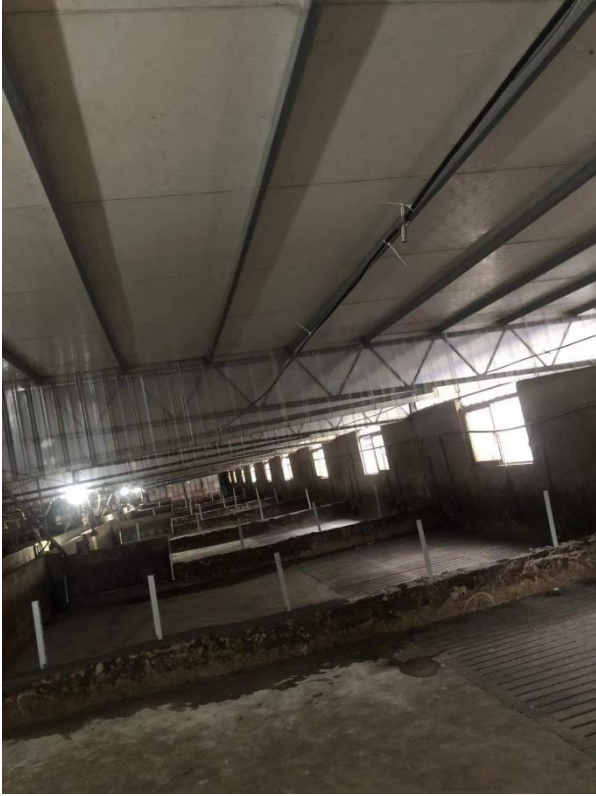
养殖场喷淋设备
