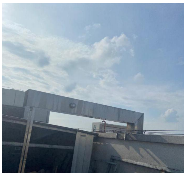
油炸废气排气筒
